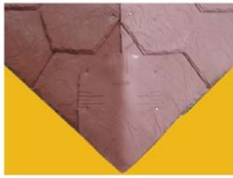
Picture 2: Install the first piece at the bottom of the hip. Cut the top shingle to line up with the other shingles. Mold shingle to the shape of the hip.
