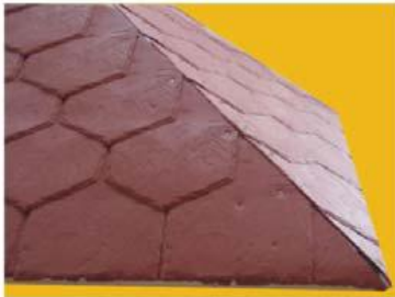
Picture 1: Install shingles on to the sides of the hip as shown above.
