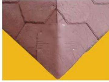
Picture 2: Install the first piece at the bottom of the hip. Cut the top shingle to line up with the other shingles. Mold shingle to the shape of the hip.
